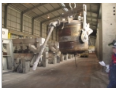
Suction pipes on collector ladle cast by Malmsteypa Thorgrims for Nordic Aluminum
