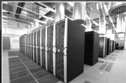
Iceland's cool climate and abundant supply of geothermal and hydroelectric energy makes it a ideal location for data centers.
